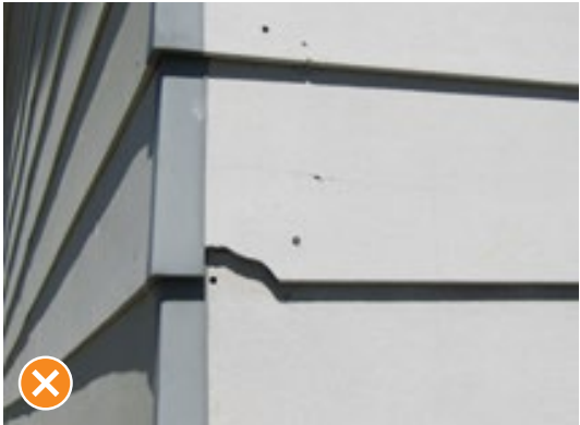
Figure 15 Damaged fibre cement weatherboard.
