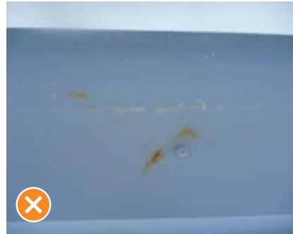
Figure 18 Rust marks on roof coating.
