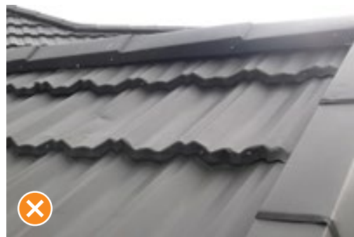
Figure 17 Dented metal tiles.
