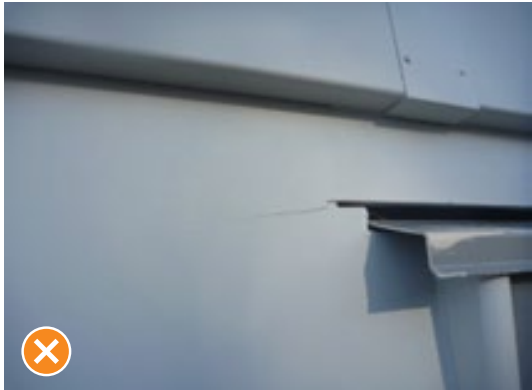
Figure 14 Crack in a fibre cement weatherboard.
